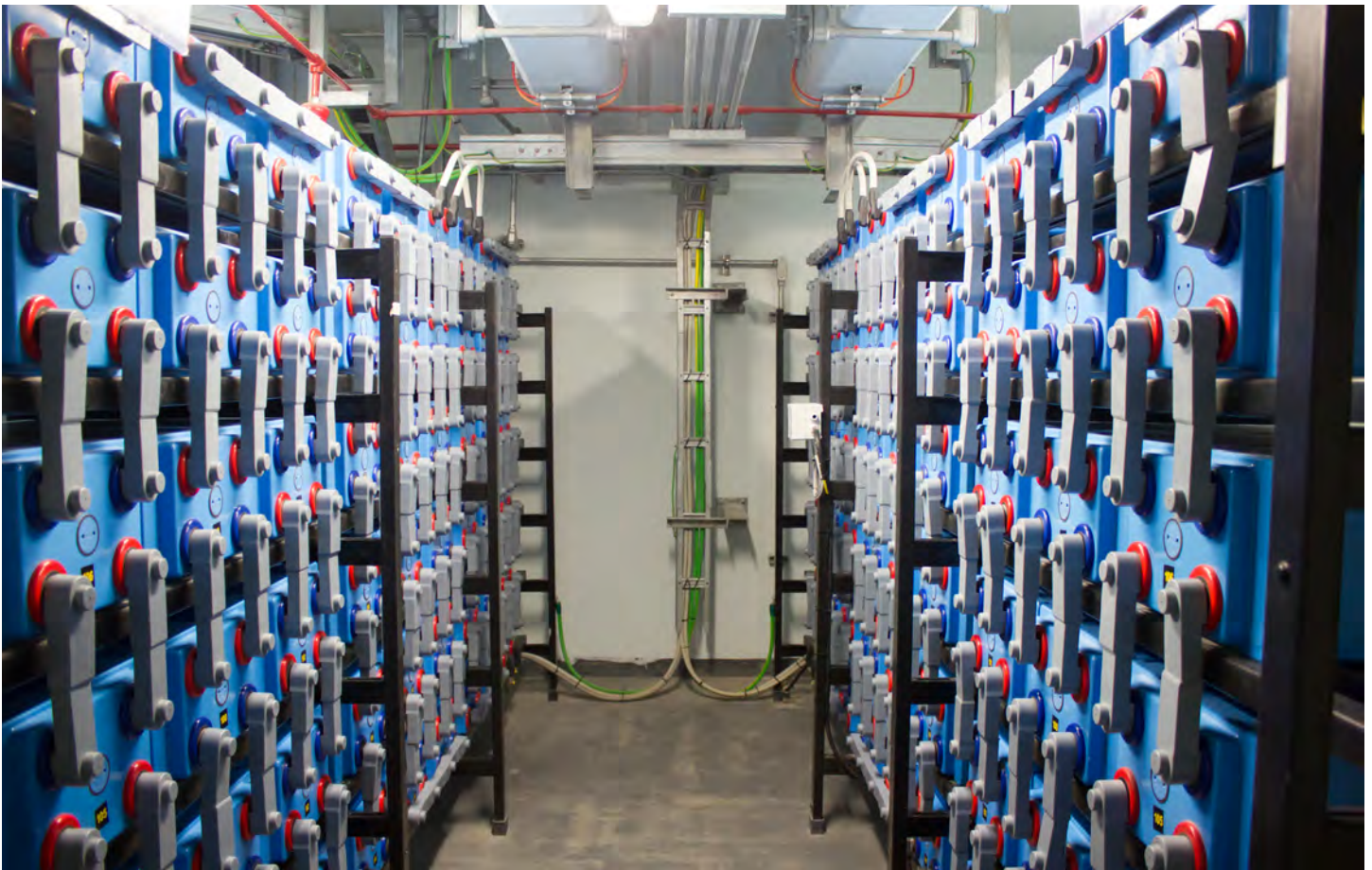
BESS are subject to thermal runaway conditions because, at their core, they utilize rechargeable batteries.
