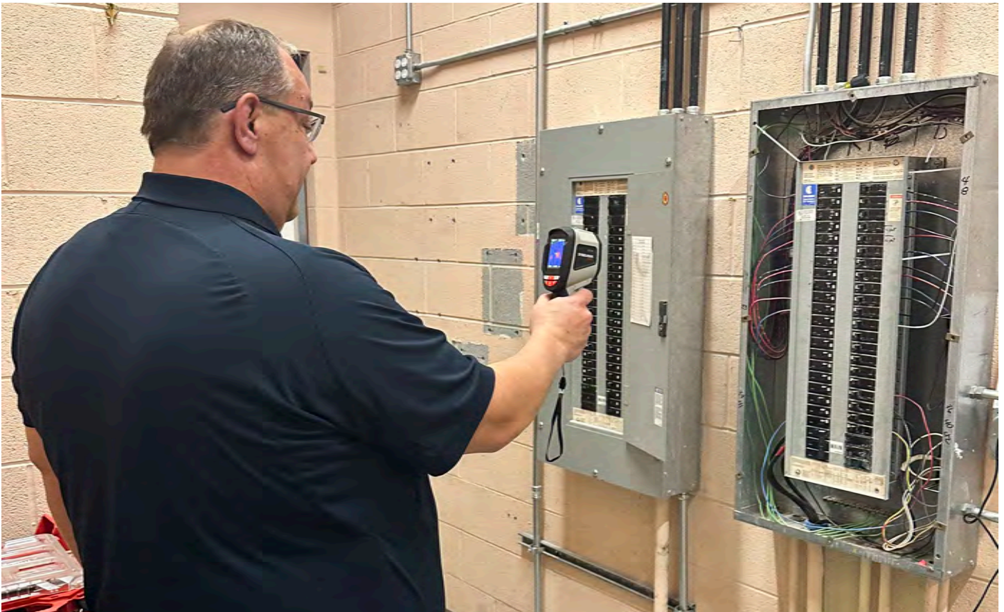
Bombard focuses on energy-efficient upgrades at CPS schools, like freon replacements, LED lighting and solar panel installs, heating system upgrades and adding electric vehicle charging stations.
