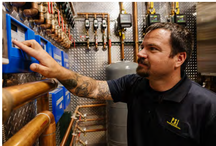
Brandon Content, at Plumbing Systems Inc., establishes a connection between several boilers and the tekmar control system that serves the large vacation home.
